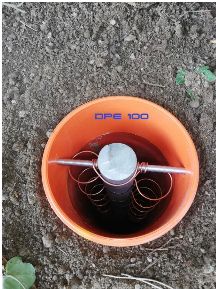
Prototype orange installé
